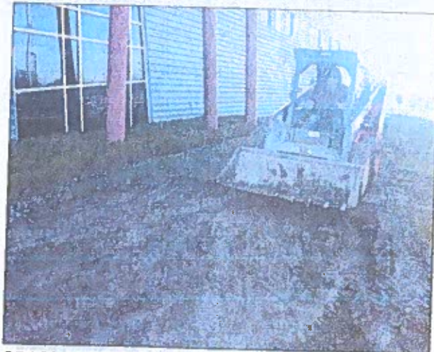
GRASS REMOVAL: Pictured is Marshall Doctor, owner of Doctor Construction, using a skid loader to remove grass at Parkview Huntington Family YMCA.
